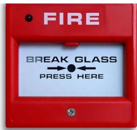
Fire alarm devices
